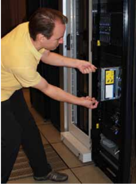
IT hardware maintenance in the computer room at BIRA-IASB.
